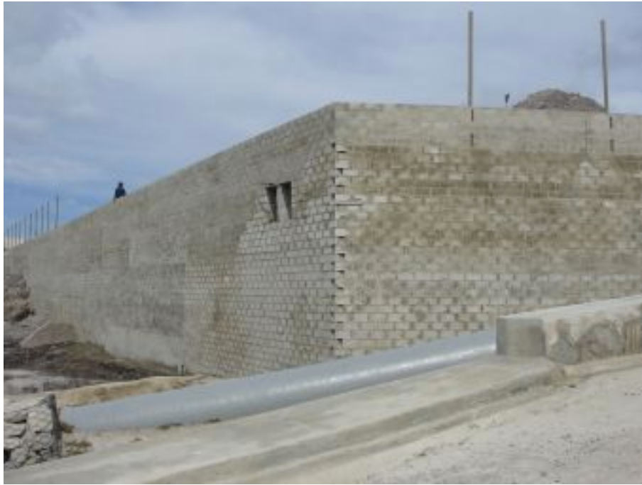
The 2m wide retaining wall completed - reaching heights of up to 12 metres in places
