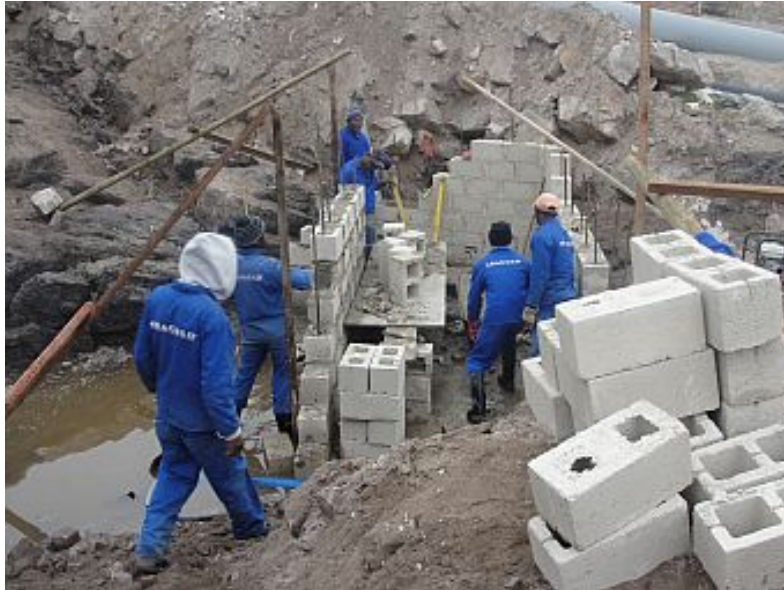
Simphiwe and his team laying the first bricks of the retaining wall
